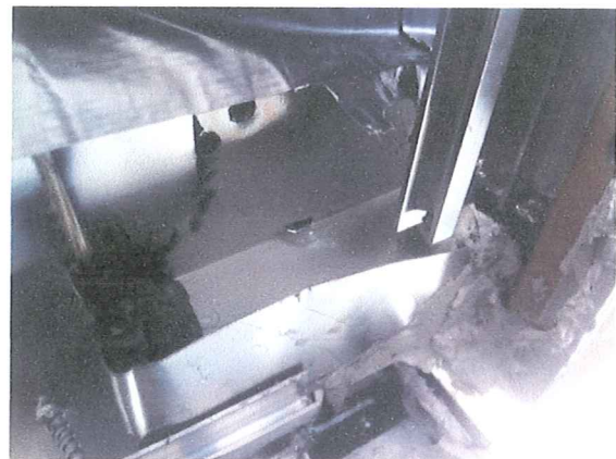
Hole in rear of head flashing
